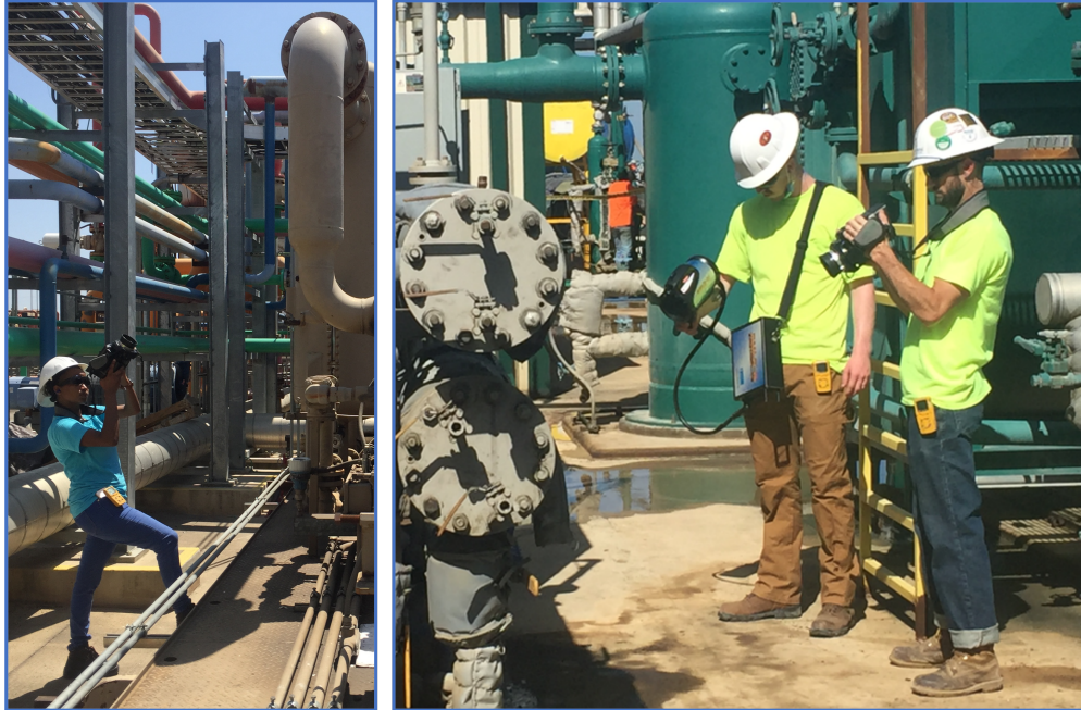
Figure 2.2: All components at the RNG plant were scanned using OGI and RMLD for methane gas detection. Identified emissions were cataloged by major equipment and component type prior to measurement.
