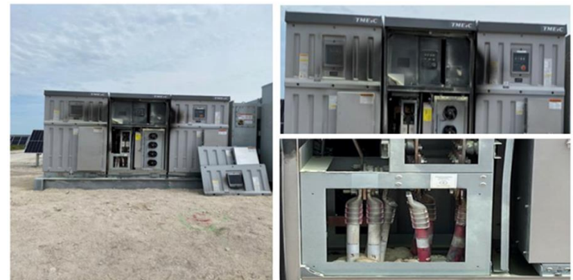
Near Miss Arc Flash – Twin Rivers Solar Project (source: Duke Energy Safety Alert , April 2021 )
