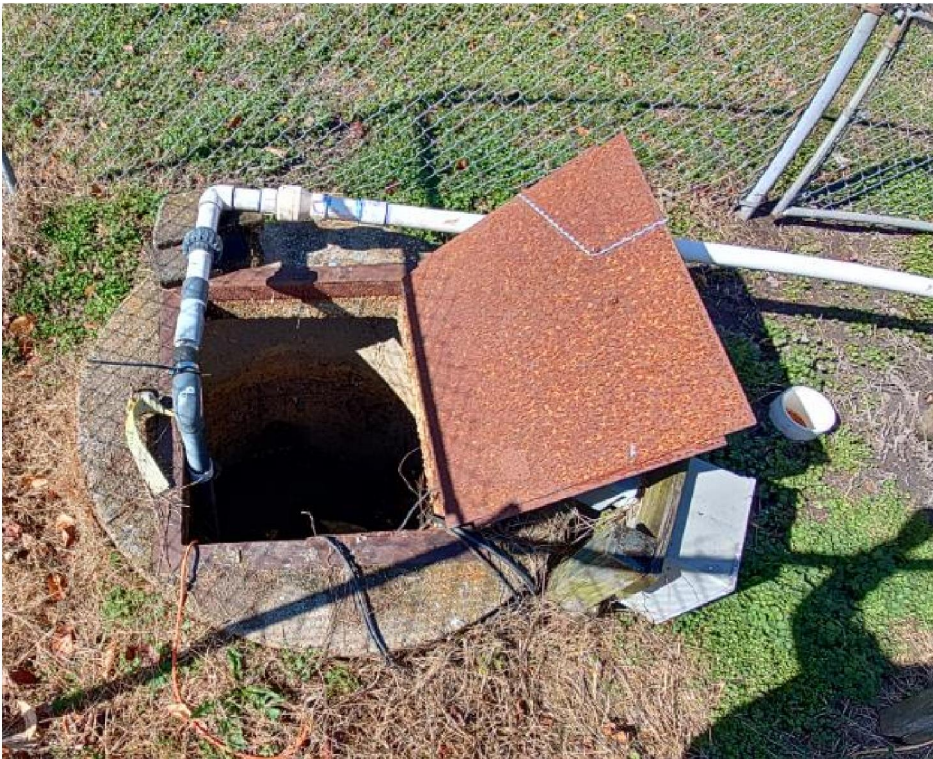
Figure 10. Universal Circle Pump Station
