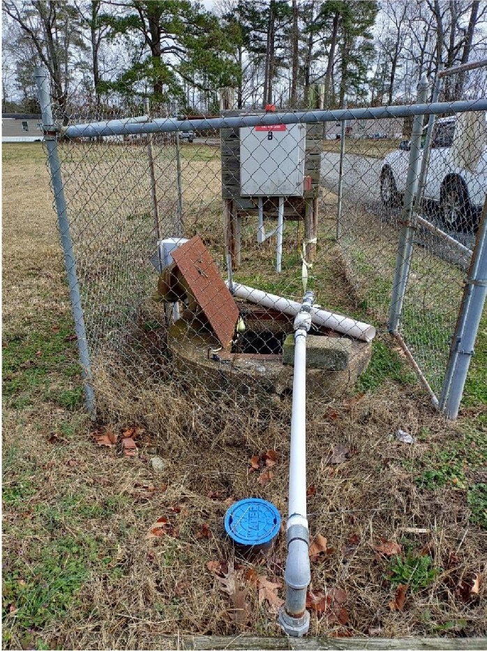
Figure 3. David Drive Pump Station
