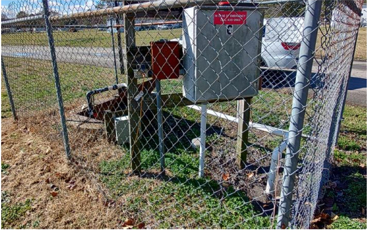
Figure 11. Universal Circle Pump Station
