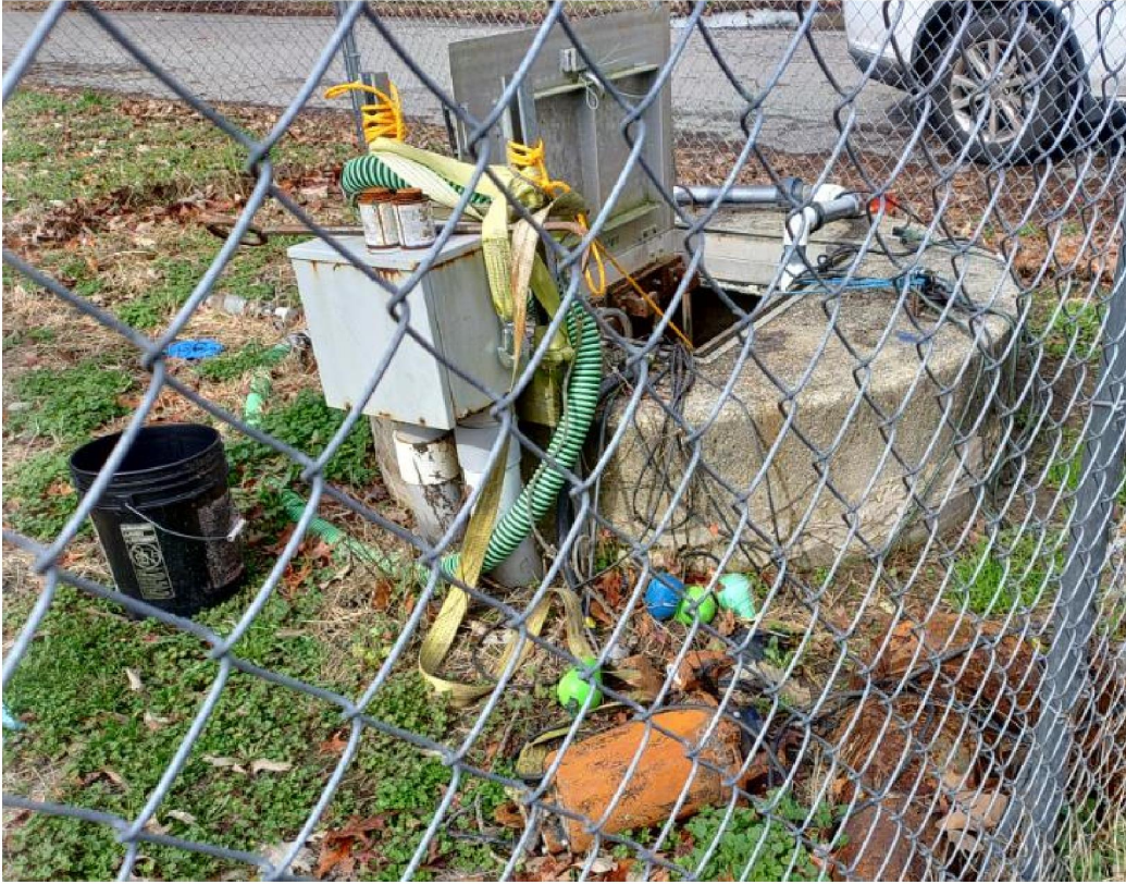
Figure 7. Perry Drive Pump Station
