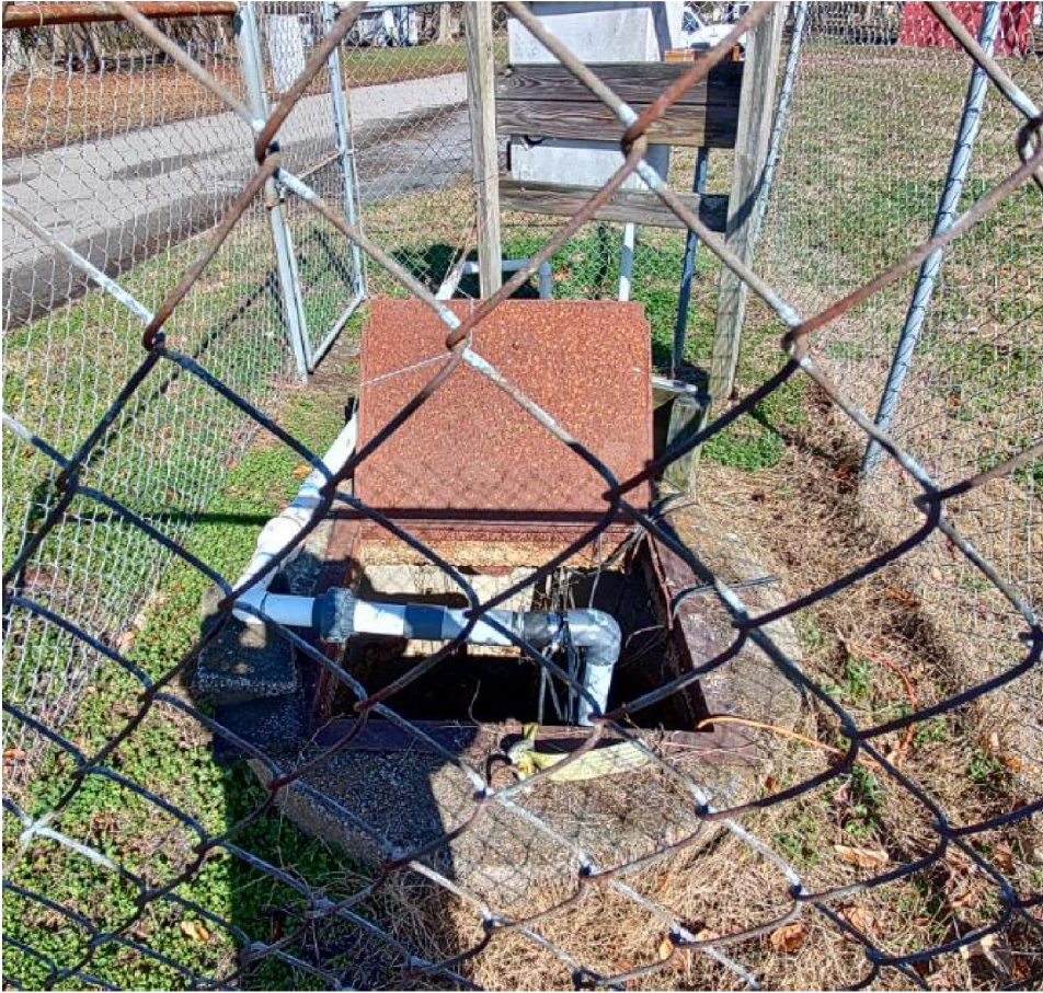
Figure 9. Universal Circle Pump Station
