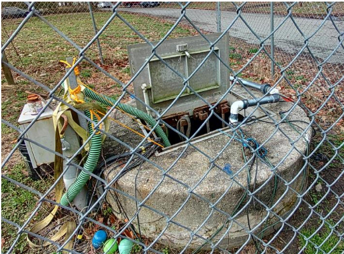
Figure 6. Perry Drive Pump Station
