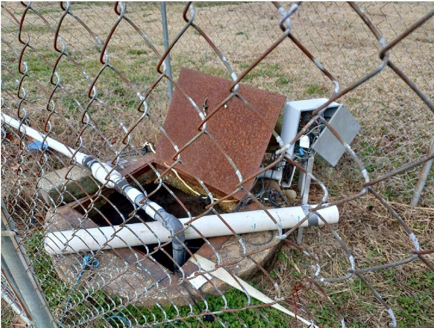
Figure 4. David Drive Pump Station
