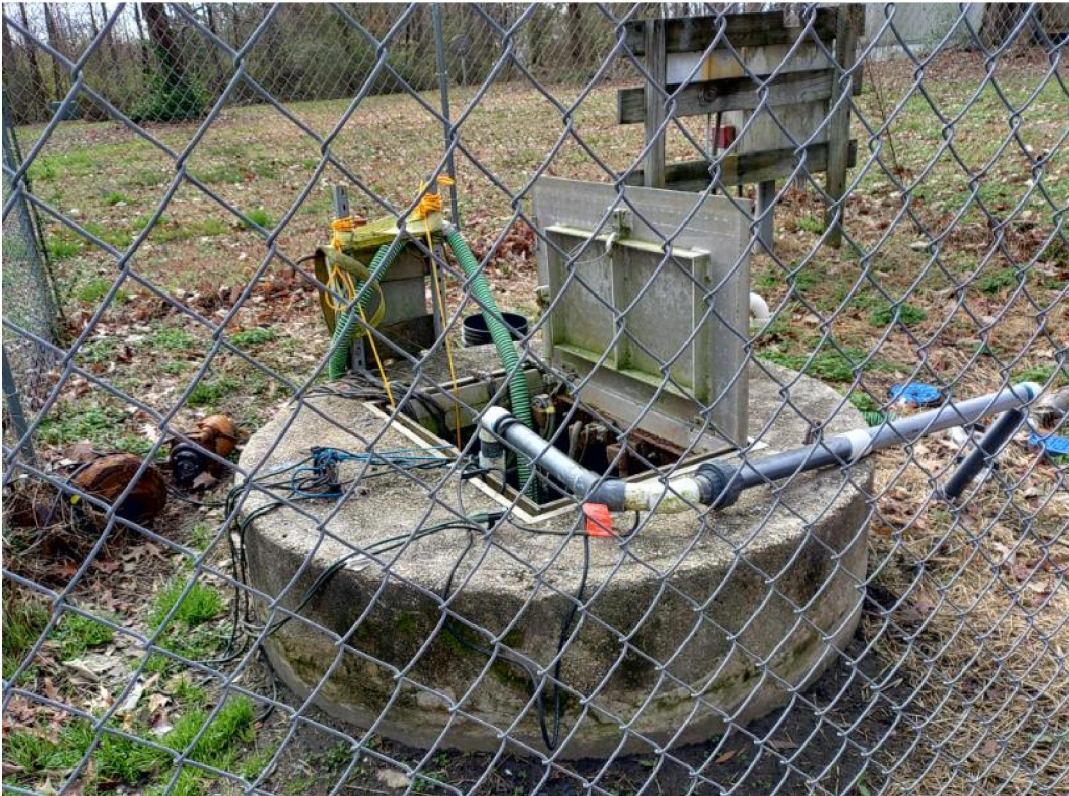
Figure 8. Perry Drive Pump Station
