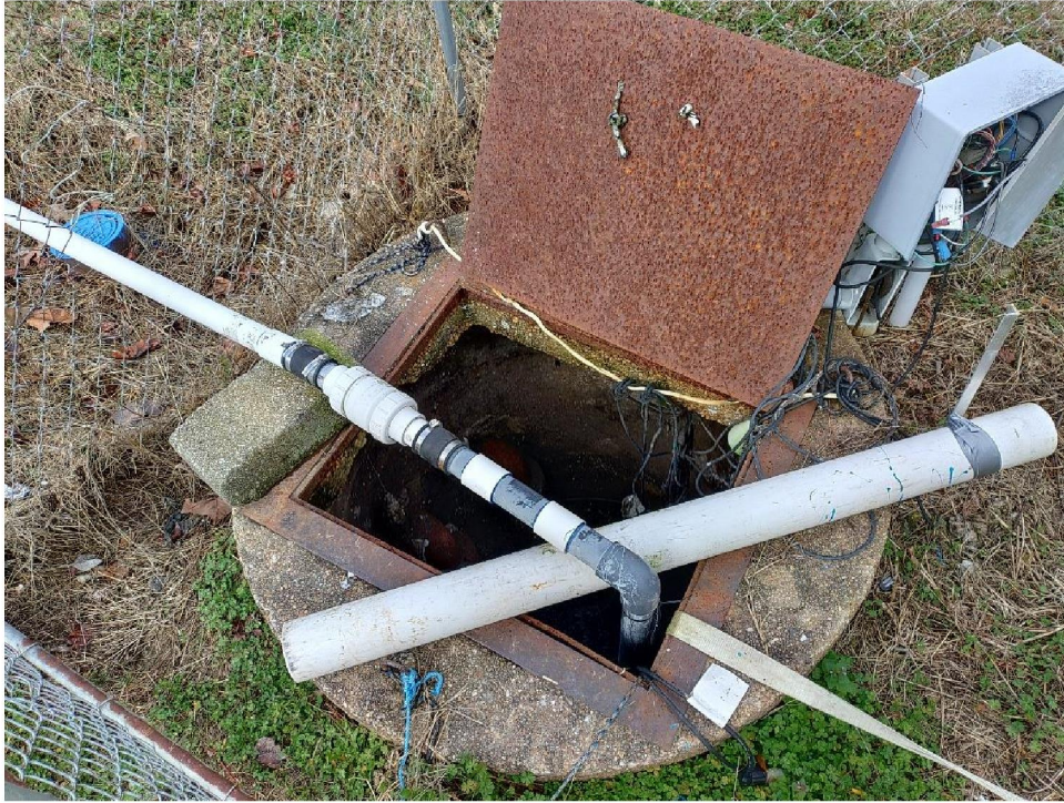
Figure 5. David Drive Pump Station
