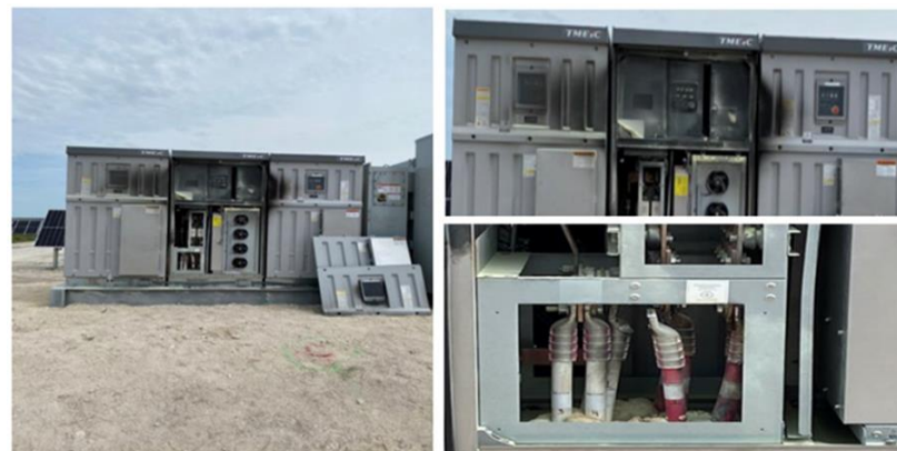
Near Miss Arc Flash – Twin Rivers Solar Project (source: Duke Energy Safety Alert , April 2021 )
