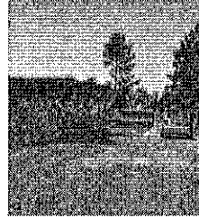
A construction crew performs shoulder work along Country Club Road in Camden County, Tuesday. Traffic was closed to one lane and an escort vehicle had to lead motorists safely past the construction work.
