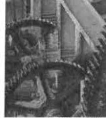
Several of the gears use to raise and lower the Camden Cousoway Bridge are seen while the bridge was raised on Saturday, Nov. 13.
