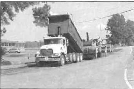
A paving project on Old Route 32 and at the intersection of Newland Road reduced traffic flow intermittently last week in Roper. The work, an NCDOT project contracted to Ross Brothers in Greenville, continues this week. [Staff photo by Dale Heberlig]
