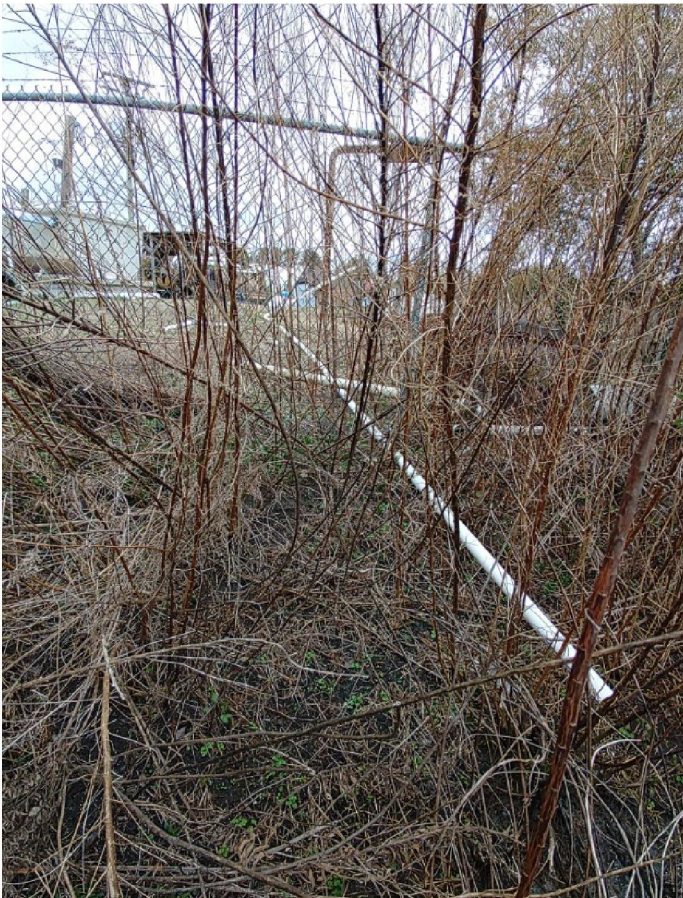
Figure 2. Unpermitted pipe for discharge of wastewater (February 13, 2024)
