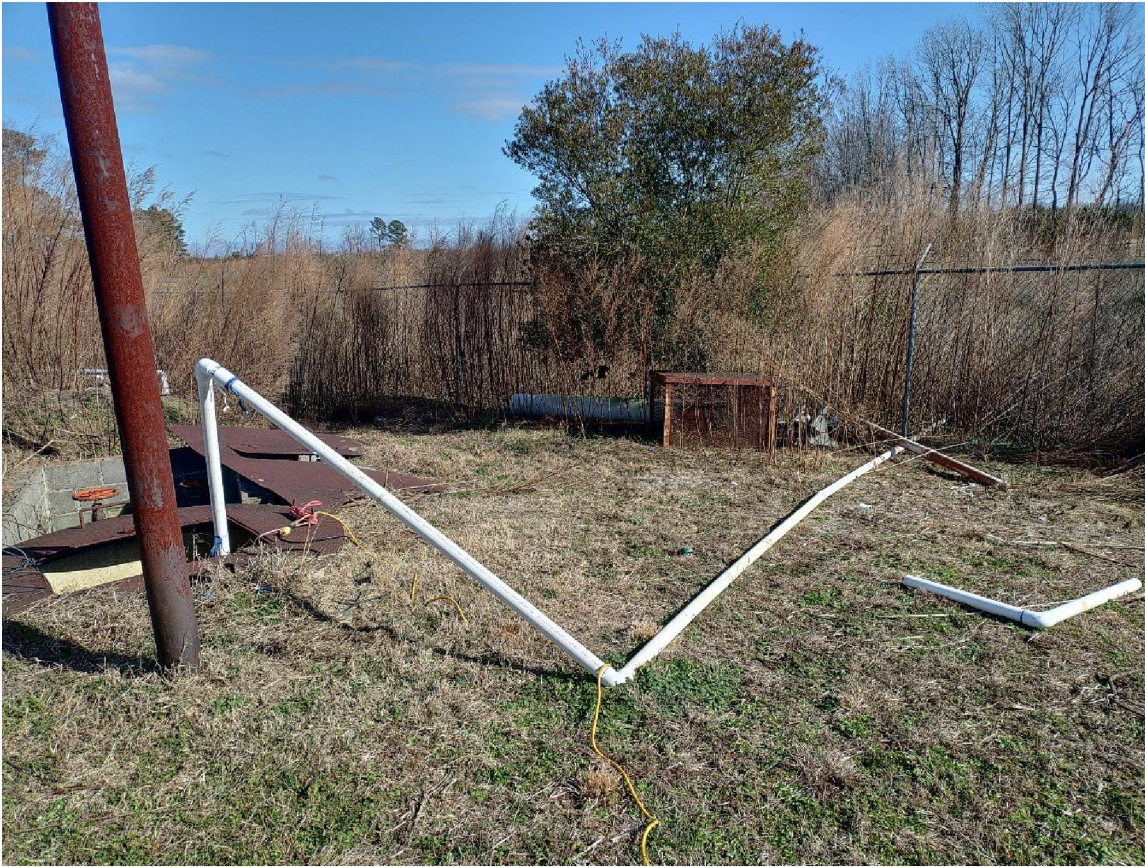
Figure 10. Unpermitted discharge (February 21, 2024)
