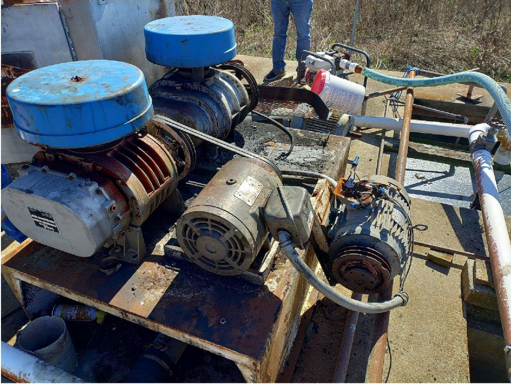
Figure 11. Inoperable blower units (February 21, 2024).
