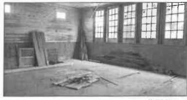
A look on the inside of the soon-to-be-transformed Rosenwald School in Hamilton.
