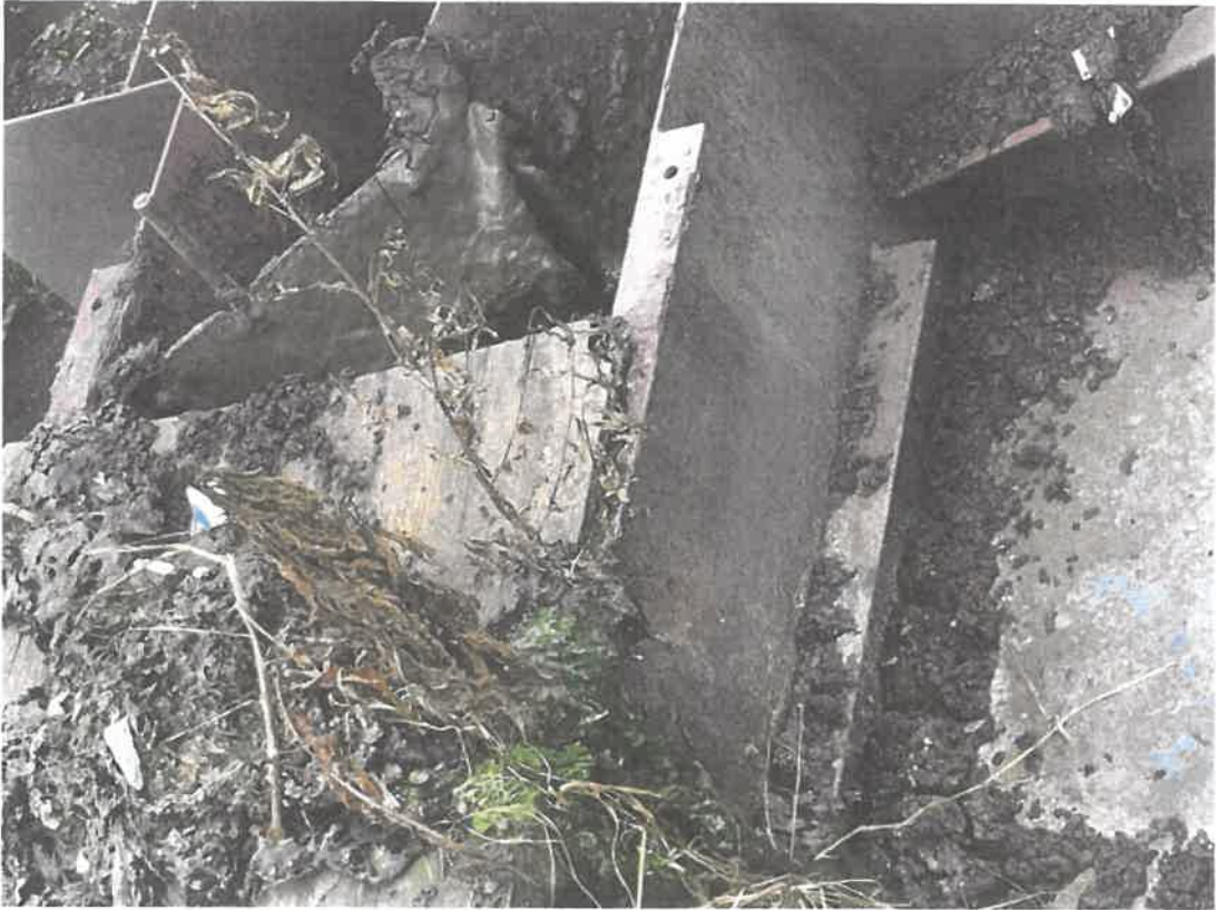
Photos: from August 4, 2020— Eagle Creek WWTP
