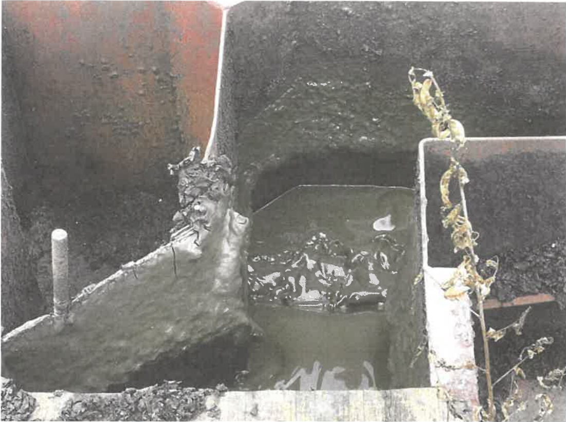
Photos: from August 4, 2020— Eagle Creek WWTP
