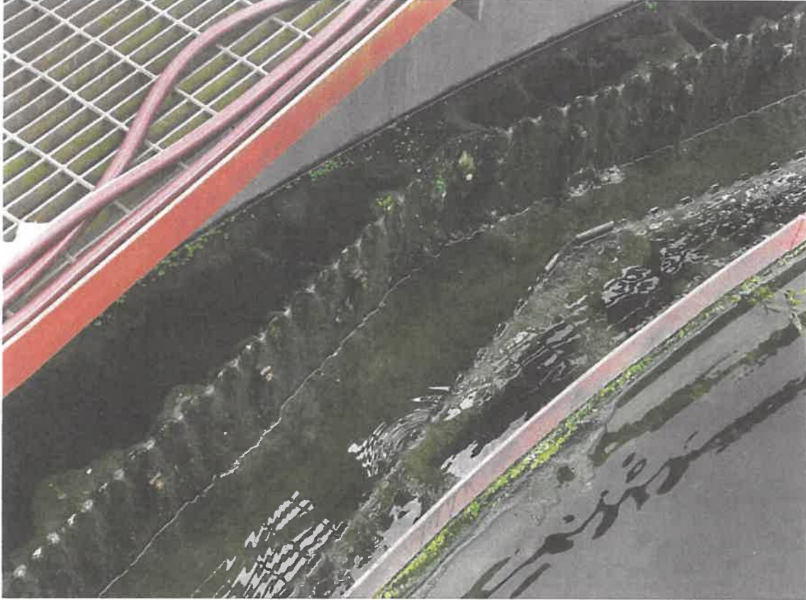
Photos: from August 4, 2020— Eagle Creek WWTP
