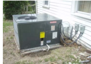
New Energy Efficient Unit
