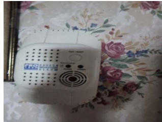
Non-Functioning CO Detector
